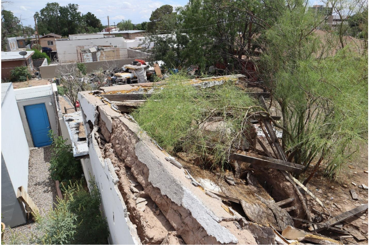
Figure 12: View of the wall to the rear of the 414 E. May property that acts as a privacy wall for the property at 422 E. May. Photo taken from the roof of 422 E. May. Photo taken July 1, 2025.
