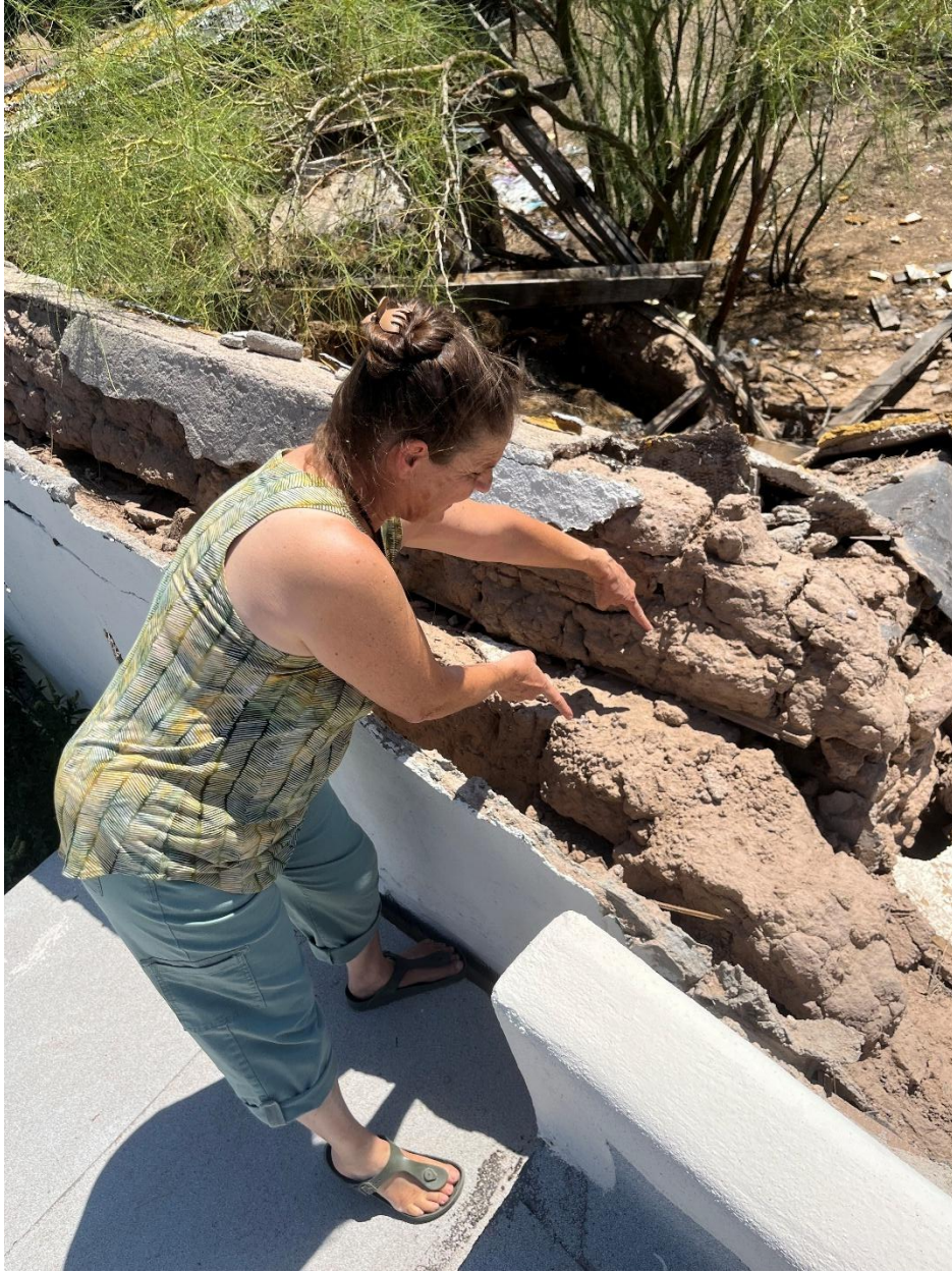
Figure 15: 422 E. May property owner and occupant Doris Buchmann illustrating how much the parapet of the roof had moved in the week between the assessments on July 1 and on July 9, following heavy rains. Photo taken July 9, 2025.
