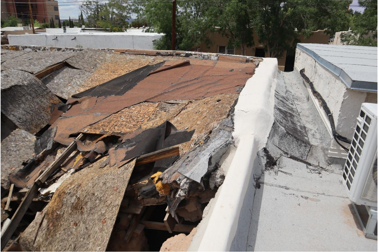
Figure 3:Roof of party wall between 422 E. May and 414 E. May. Photo taken July 1, 2025.
