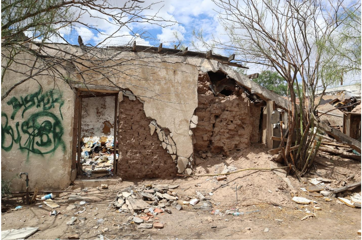
Figure 7: Condition of south façade of property, with collapsed ceiling and roof structure. Photo taken July 1, 2025.
