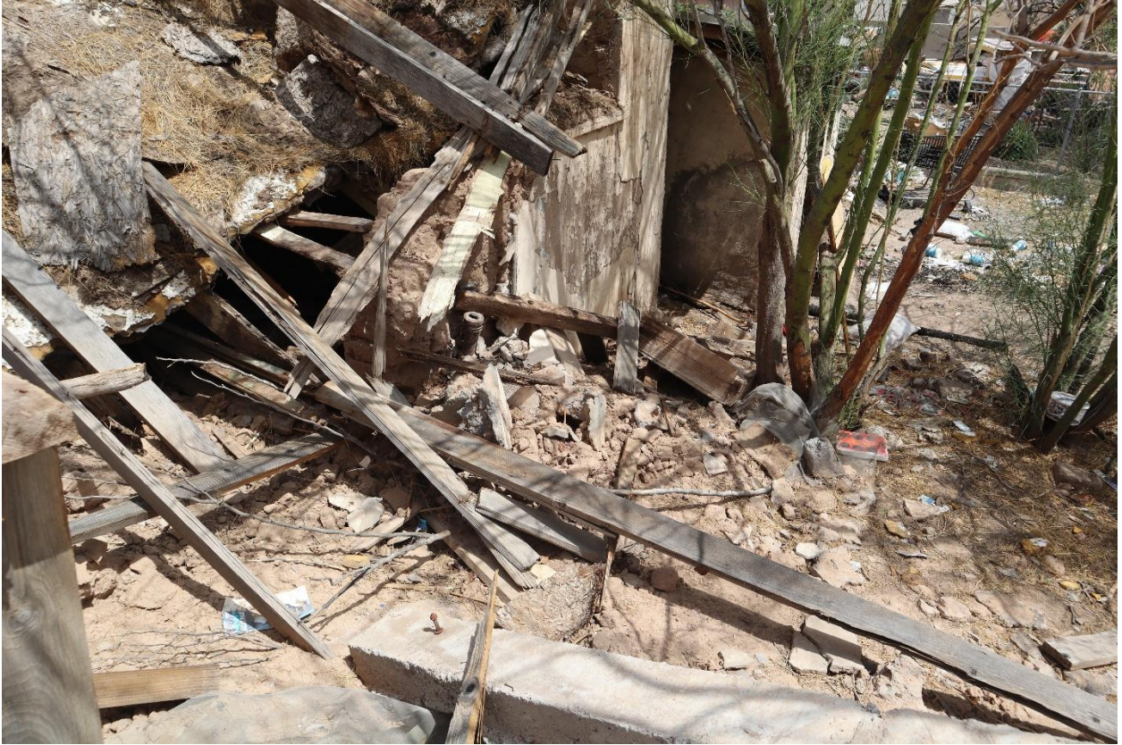
Figure 10: Detail of collapsed roof and wall structure. Photo taken July 1, 2025.
