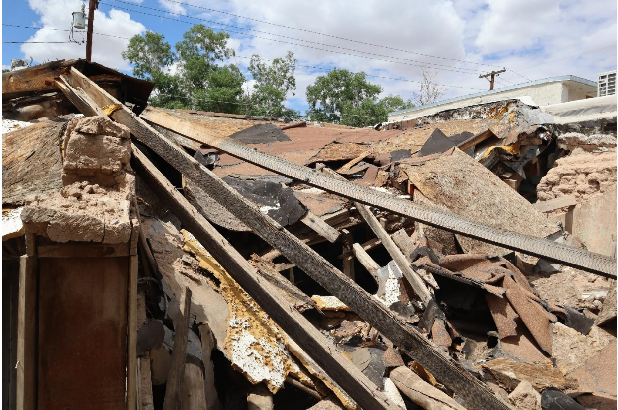
Figure 9: Detail of collapsed roof and wall support structure. Photo taken July 1, 2025.
