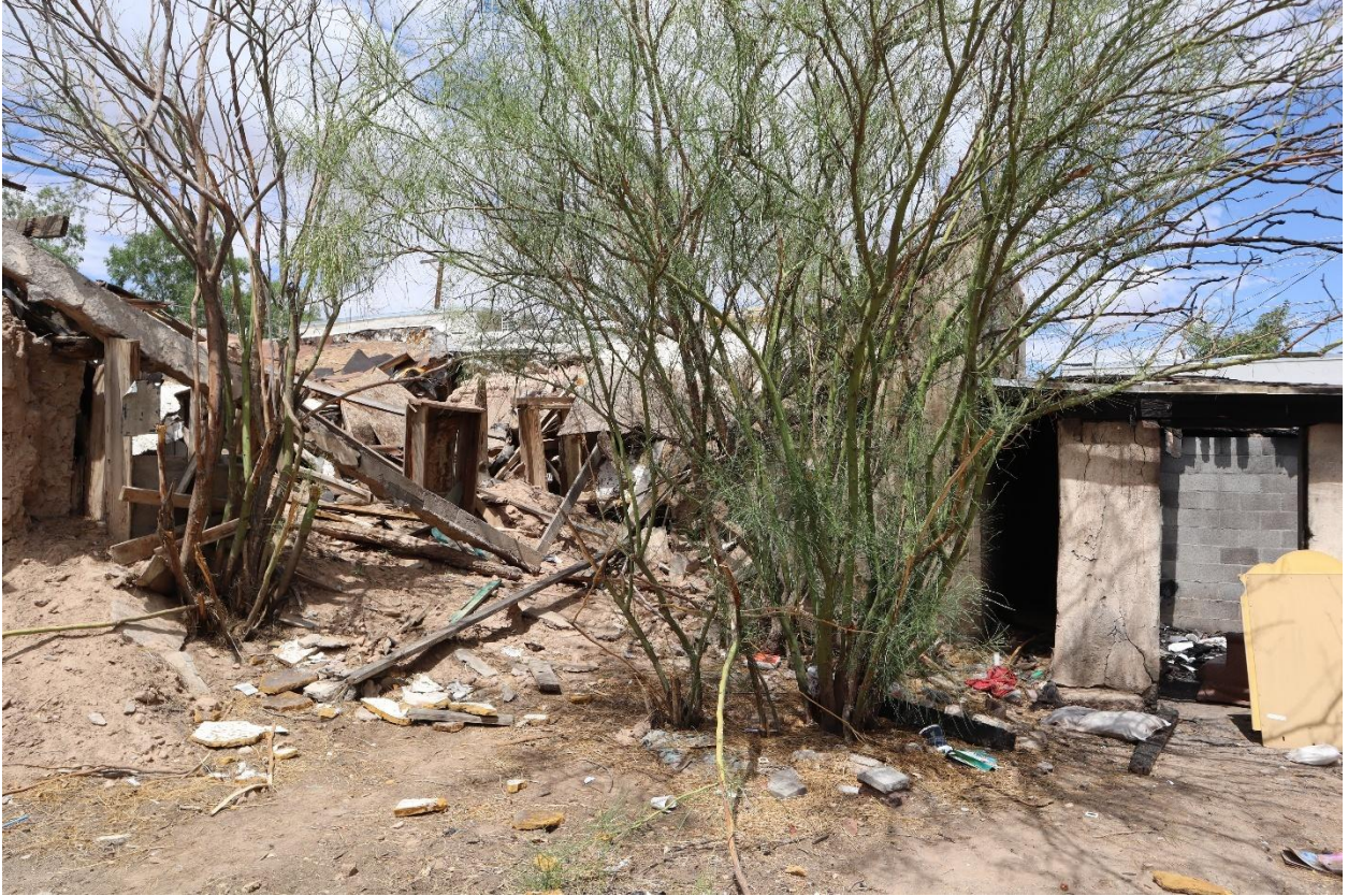
Figure 8: Collapsed roof and melted adobe mix on south façade of property. Photo taken July 1, 2025.
