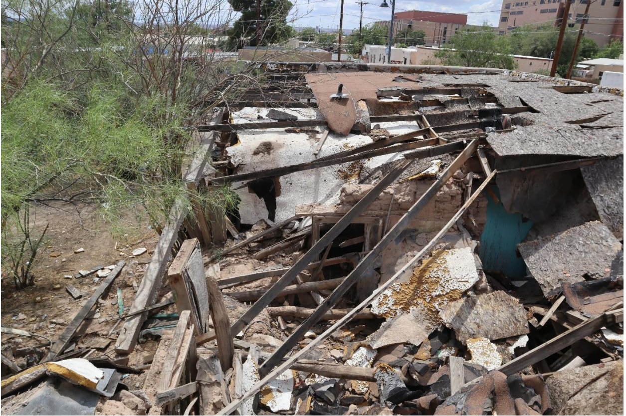
Figure 13: Photo of Collapsed roof, south facade at 414 E. May. Photo taken July 1, 2025.
